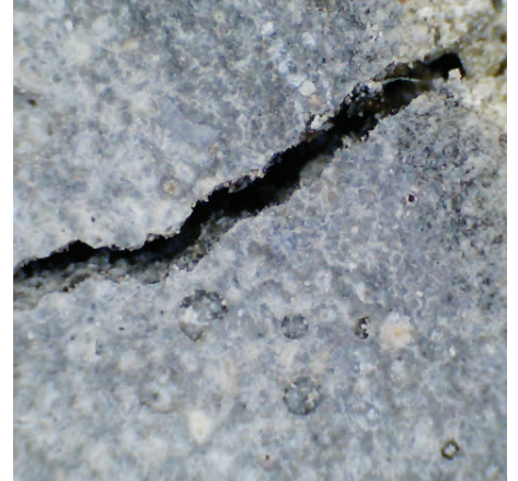
Concrete beam without AQUAFIX (0.5 mm crack)
